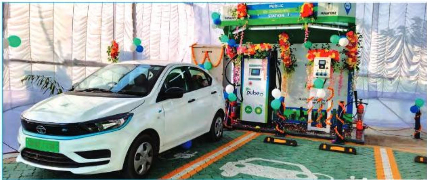
EV Charging Station
