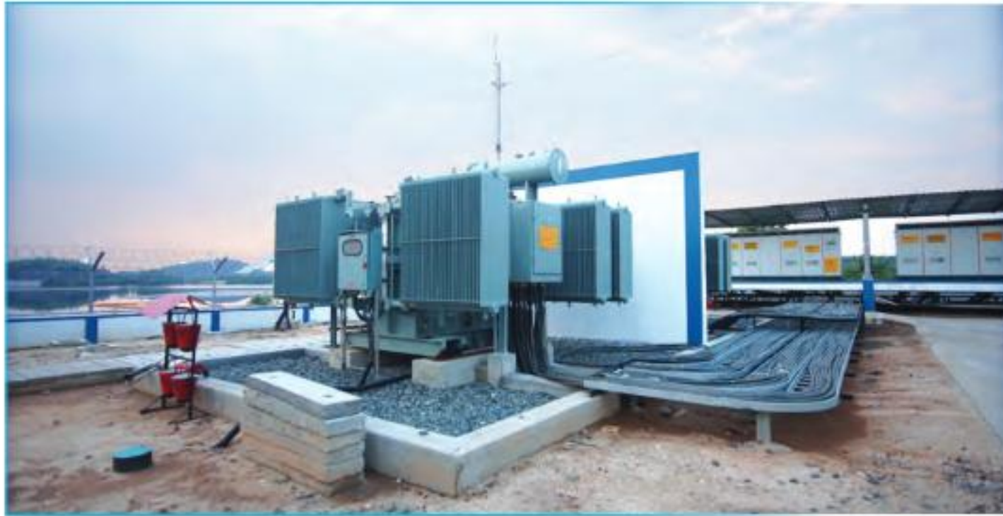
PPSP 10MW Floating SPV
